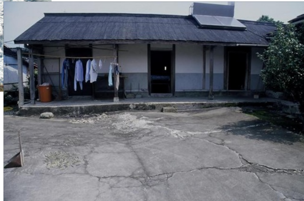
Fault creeping Chihshang in Taitung
